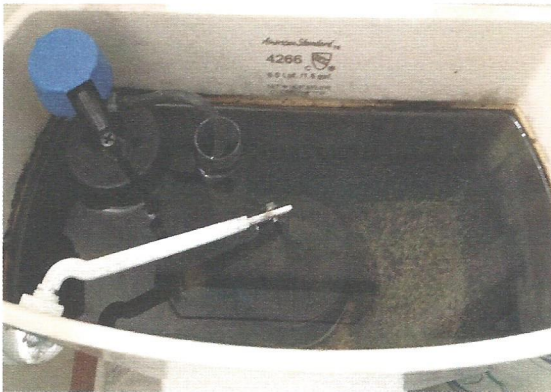
Figure 1. Mn-oxide formation in a toilet tank
